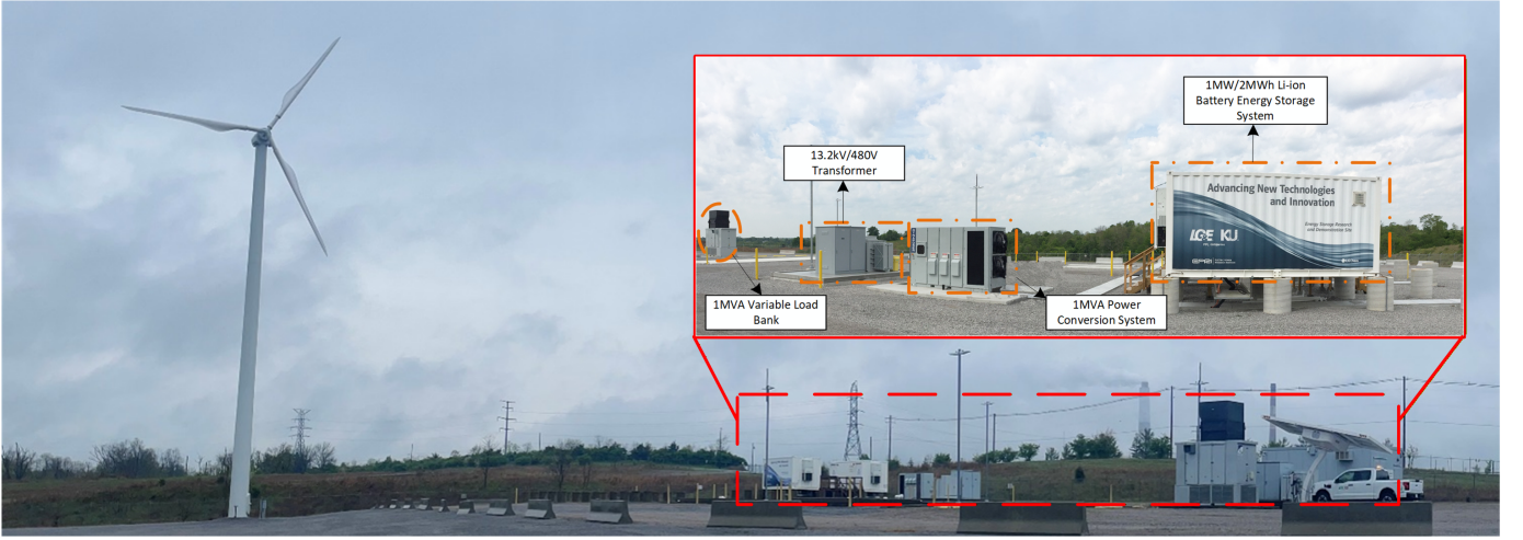
Fig. 1. Experimental setup at the PPL Renewable Energy Integration Research Facility, located at the E.W. Brown Generation Station. The site integrates a utility-scale wind turbine, a 1 MW/2 MWh Battery Energy Storage System, and a utility-scale solar PV array for renewable generation and grid-integration studies. The inset highlights the BESS installation, including the power conversion system, variable load bank, and 13.8kV/480V transformer configuration.
