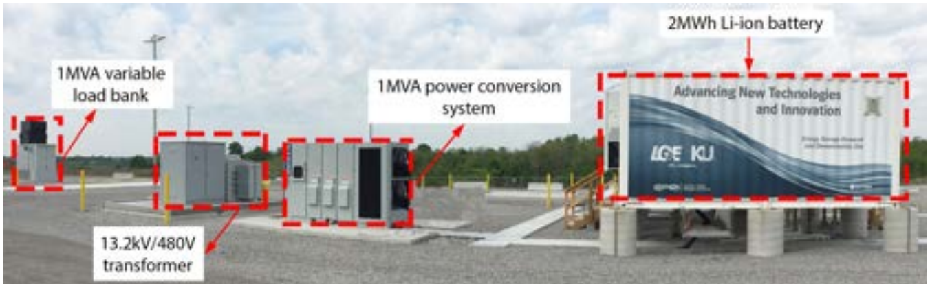
FIGURE 1. An example battery energy storage system (BESS) setup including a 1MVA bidirectional inverter, 2MWh battery system distributed in two containers (one obscured by the other), and an advanced SCADA facility, which is not shown. The 2MWh battery system incorporates 4,760 cells (20 racks or 340 modules) connected in series and parallel to meet power conditioning devices requirements.
