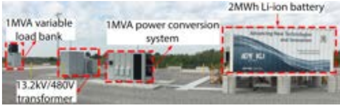
Fig. 1. The 1MVA/2MWh battery demonstrator unit installed at the LG&E and KU E.W. Brown universal solar facility as a joint project with EPRI employed for this study.
